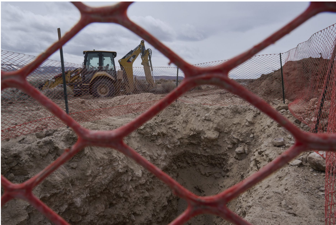
Construction has begun at the Lithium Americas project with GM at Thacker Pass in Nevada.
